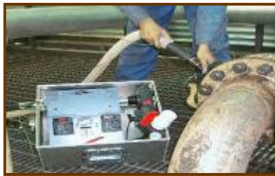
Oil and Gas Systems
